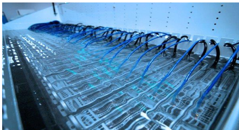
DATA Centre Cooling
