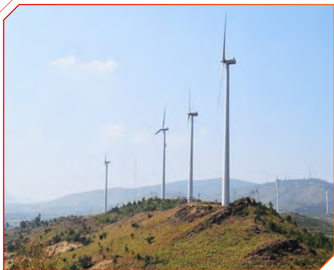
4X950kW Wind Power Project at Chitradurga, Karnataka
