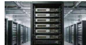
AI_HPC Server Rack
