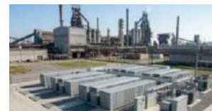
BESS for Industrial Application
