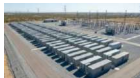
Grid Scale BESS
