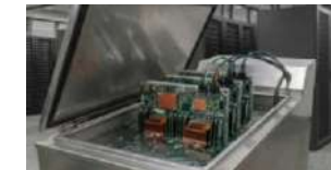
Immersion Cooled Data Centre
