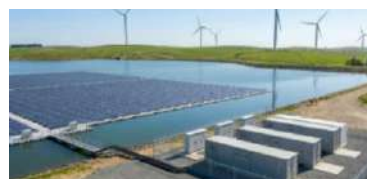
BESS for Renewable Energy Integration
